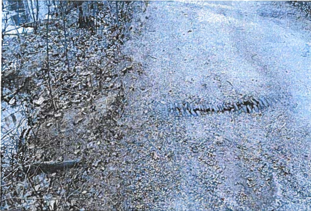
Photo 2... Westerly view showing crushed corrugated plastic pipe in driveway.
