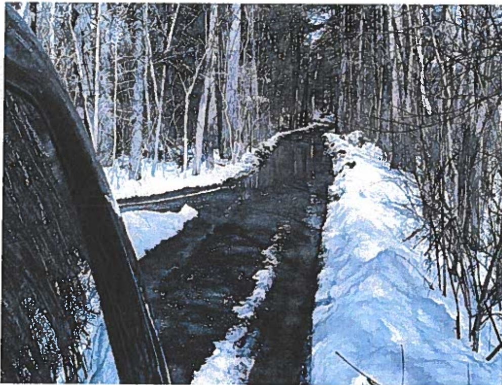
Photo 1...Easterly view showing pot-holes in gravel driveway.
