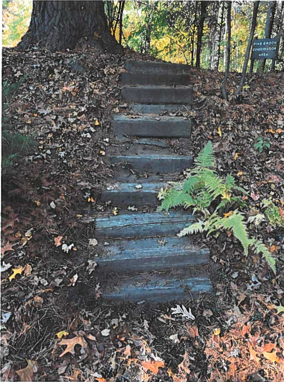
Existing stairs at the Pine Brook entrance. Rebar is sticking out of the wood, and the stairs are unsafe to walk on.
