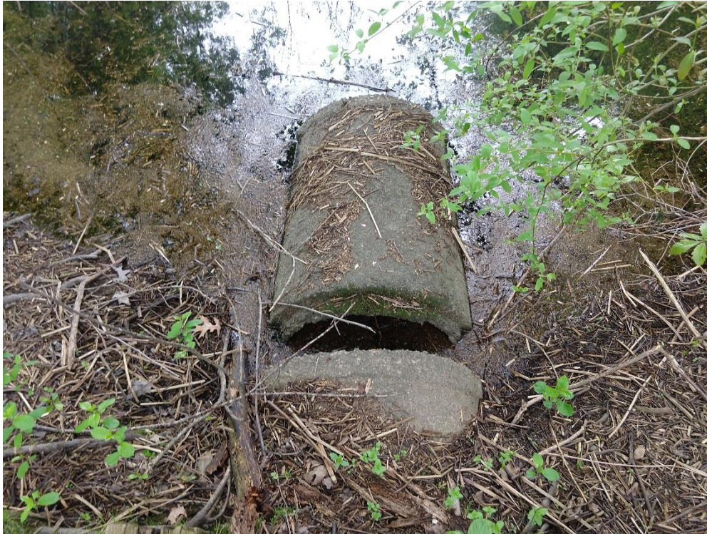
Figure 15: Culvert in need of repair along Western boundary on Bay Circuit Trail. Located on trail between southern field and community gardens.
