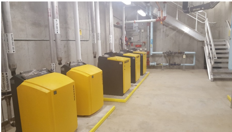
An inside look at the wastewater treatment plant.
