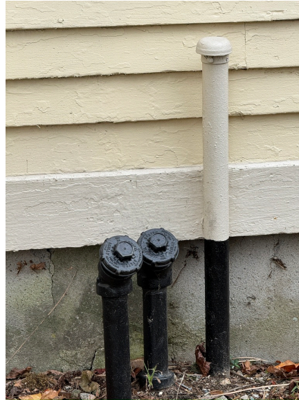
Exterior – capped pipes to fill oil burners
