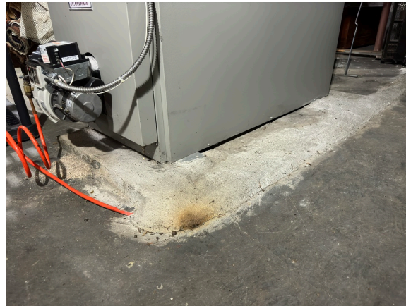
Basement – oil burner – north (right) side
