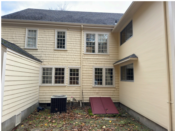
Rear elevation of main block – Willy's shed to left – 1964 addition to right
