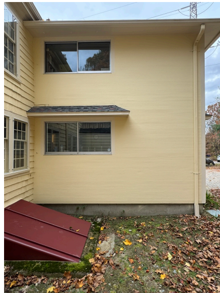
GHM – South elevation of 1964 addition – likely site of exterior part of heat pump
