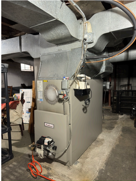
GHHM – Basement – oil burner and duct work – looking west, southwest
