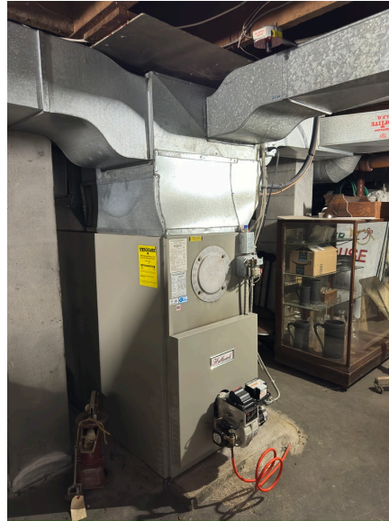
Basement – oil burner and duct work – looking west, northwest
