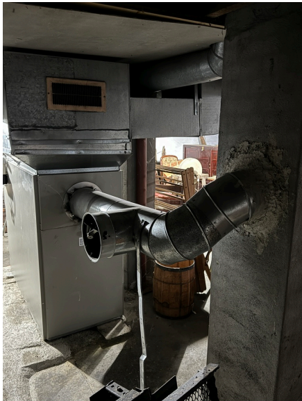
Basement – oil burner rear view – looking east, southeast
