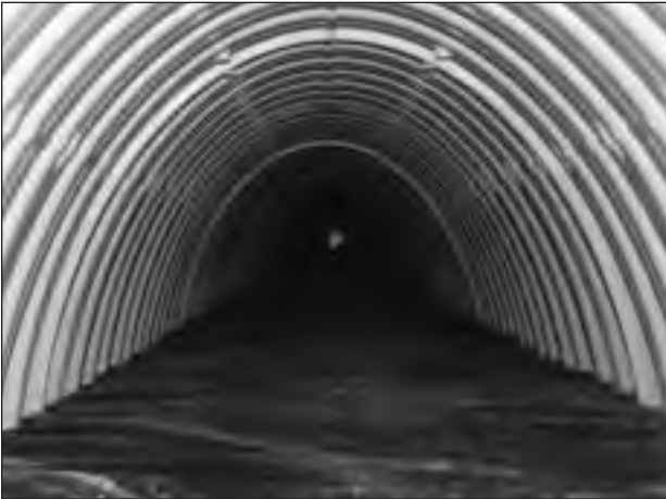
Looking down the Isolator Row from the manhole opening, woven geotextile is shown between the chamber and stone base.
