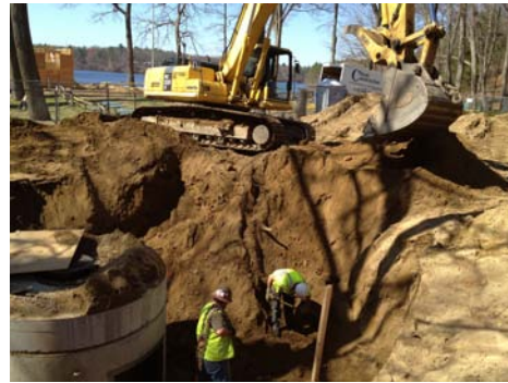
Town Beach Stormwater Separator
