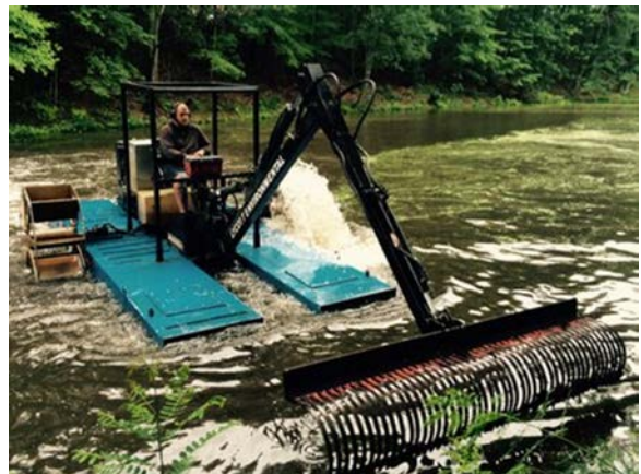
Mill Pond Hydro Raking
