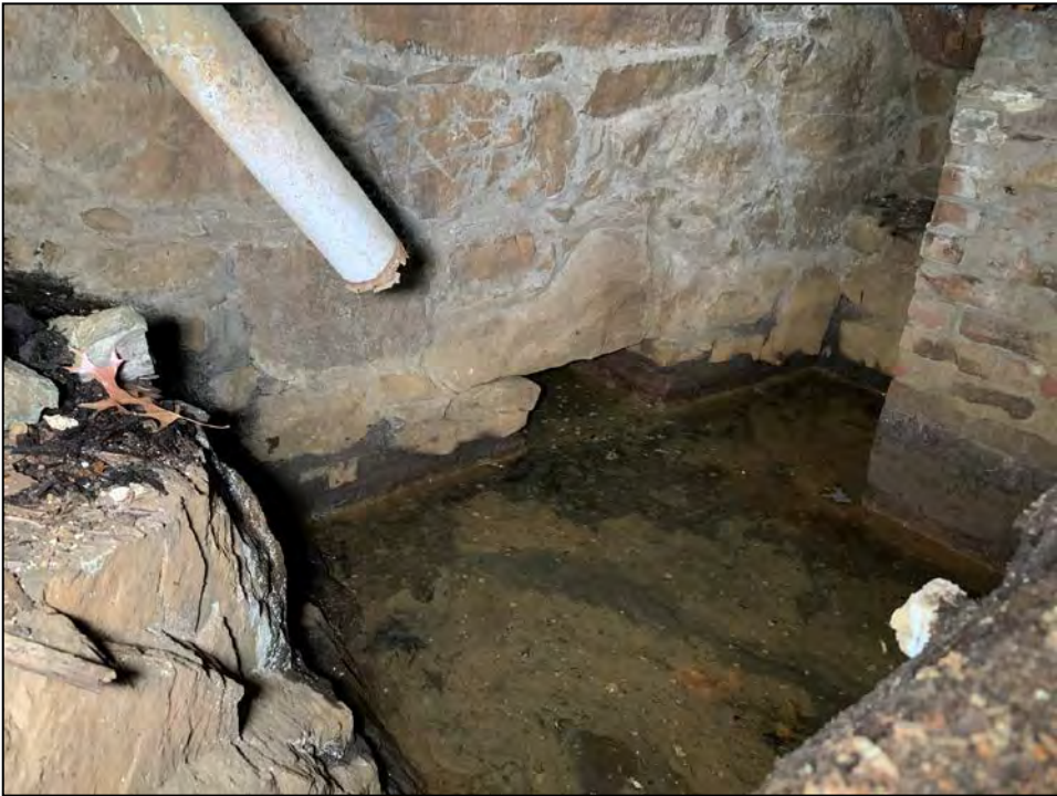
Photo No. 21: Outlet culvert in the base of the downstream wall of the gatehouse.
