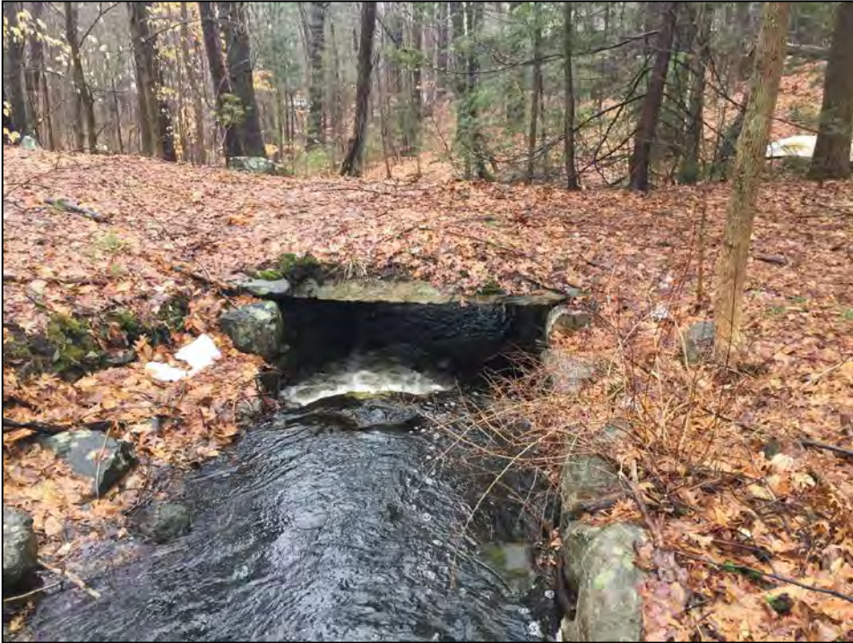
Photo No. 15: Stone culvert that carries the spillway channel beneath the crest.
