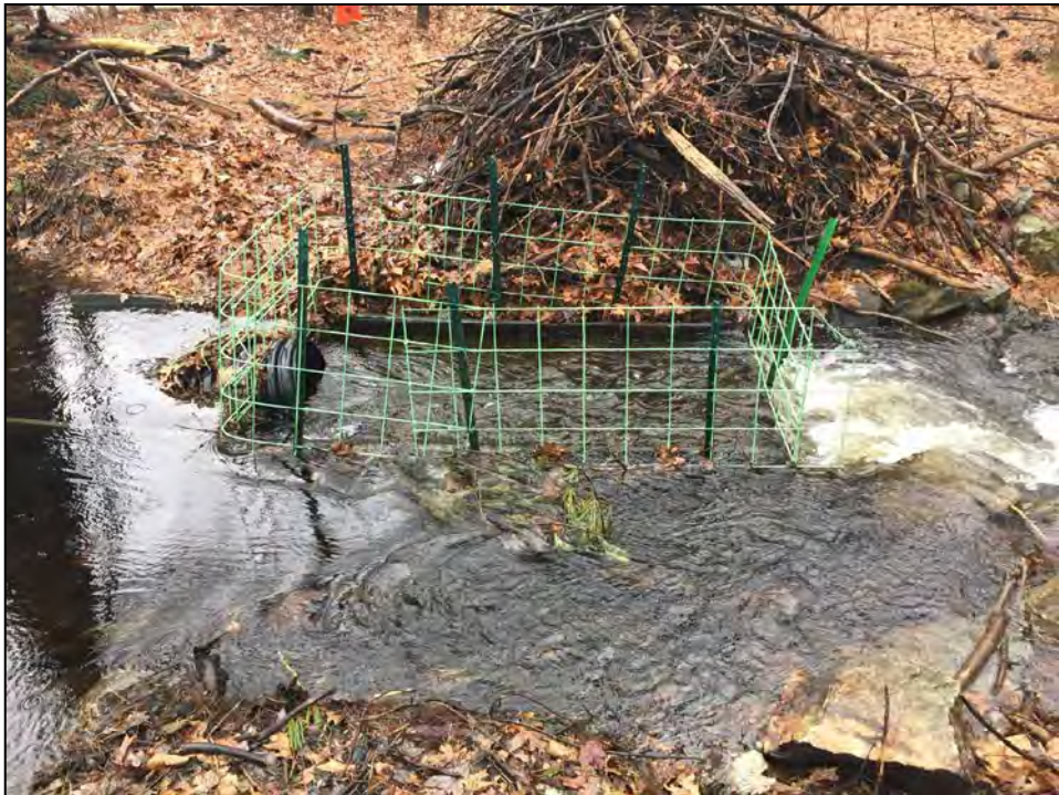
Photo No. 12: Spillway control section with apparent past beaver deceiving devices.
