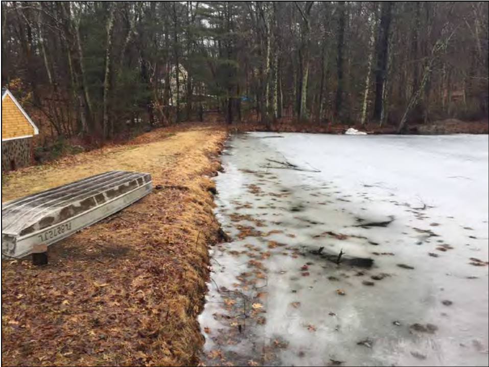
Photo No. 3: Upstream slope from the left abutment looking right. Note limited freeboard at the dam.
