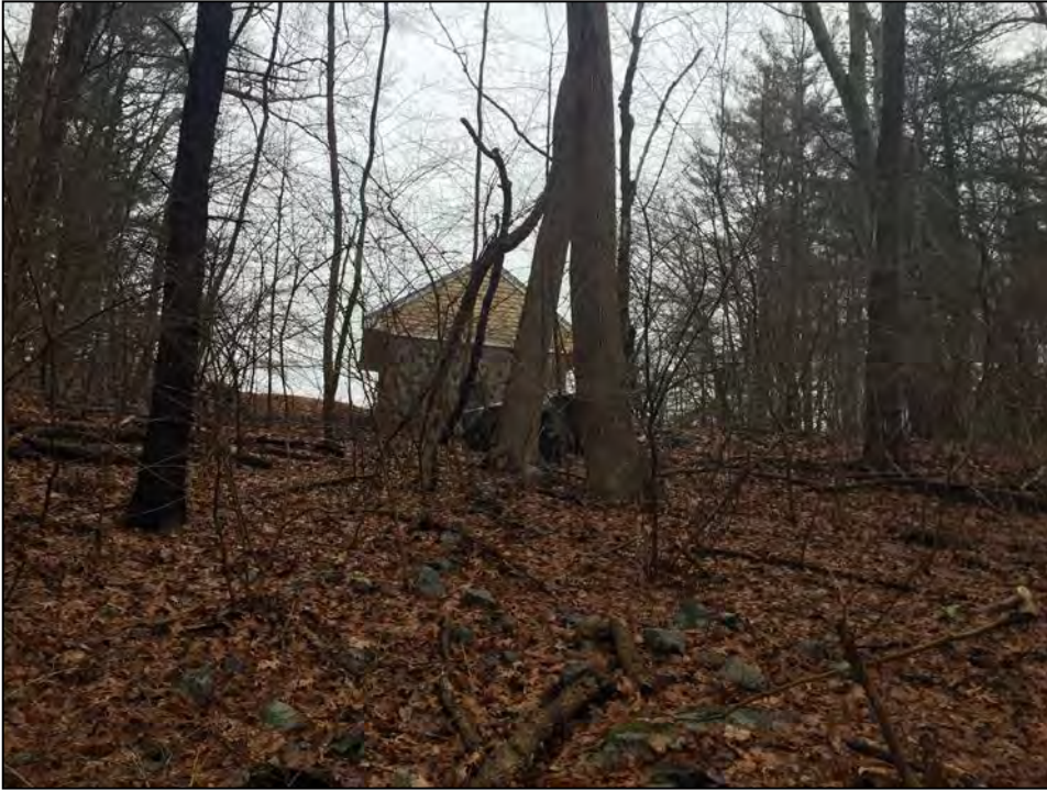
Photo No. 25: Ground surface along alignment of outlet culvert from the outlet end of the culvert looking upstream.
