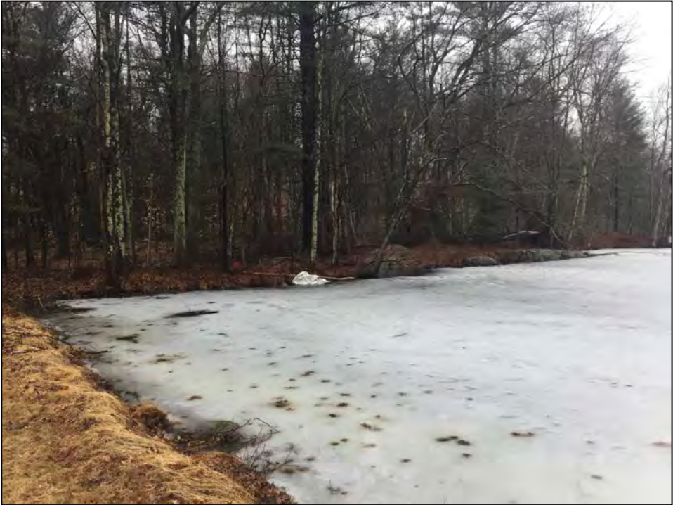
Photo No. 9: Spillway approach from the dam crest looking upstream and right..
