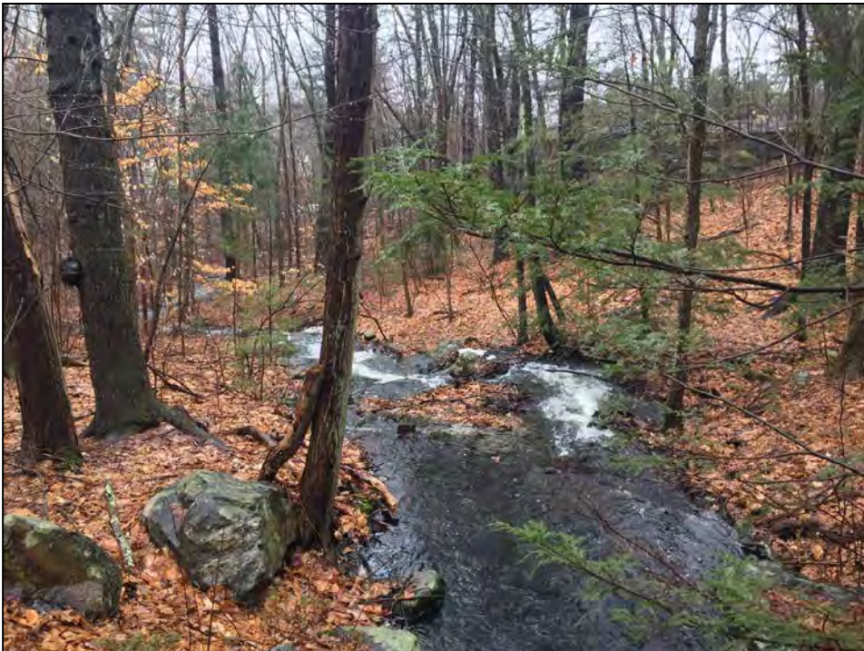
Photo No. 16: Discharge channel of the spillway from the stone culvert looking downstream.
