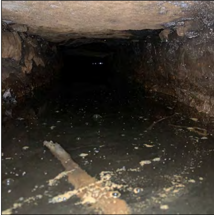
Photo No. 23: Outlet culvert interior from the upstream end at the gatehouse looking downstream. Note daylight at the downstream end of the culvert at the downstream channel.
