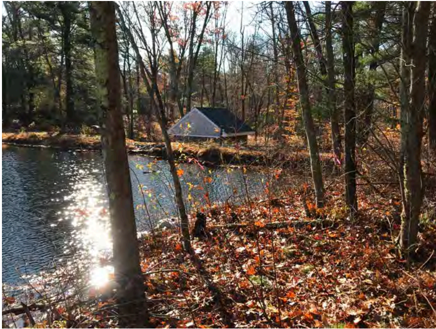
Photo 3: Wooded section of bank at upstream right side of dam, facing southeast toward gatehouse.
