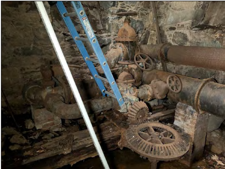
Photo No. 20: Overview of the water supply piping from the upstream left corner of the gatehouse looking looking downstream and slightly right.
