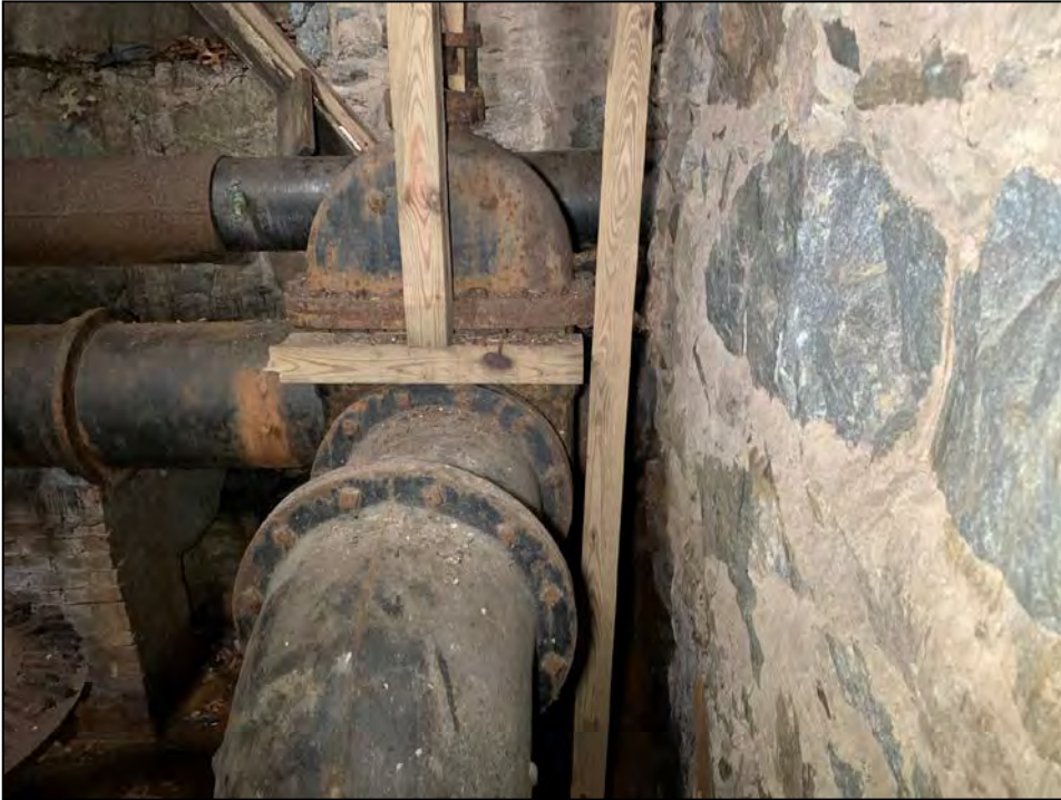
Photo No. 19: Intake lines extending through the upstream wall of the gatehouse.
