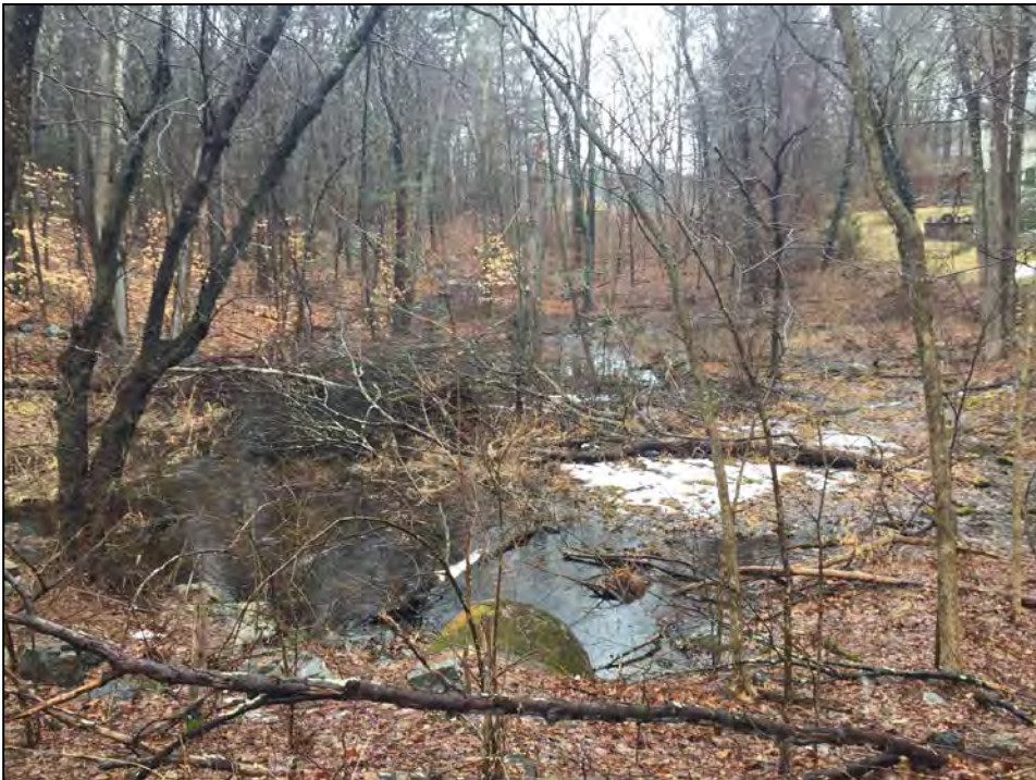
Photo No. 28: Downstream channel from the Woodbridge Road culvert crossing looking upstream.
