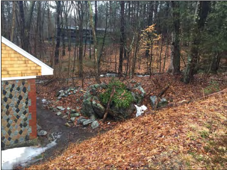
Photo No. 8: Apparent bedrock outcrop in the downstream slope right of the gatehouse.
