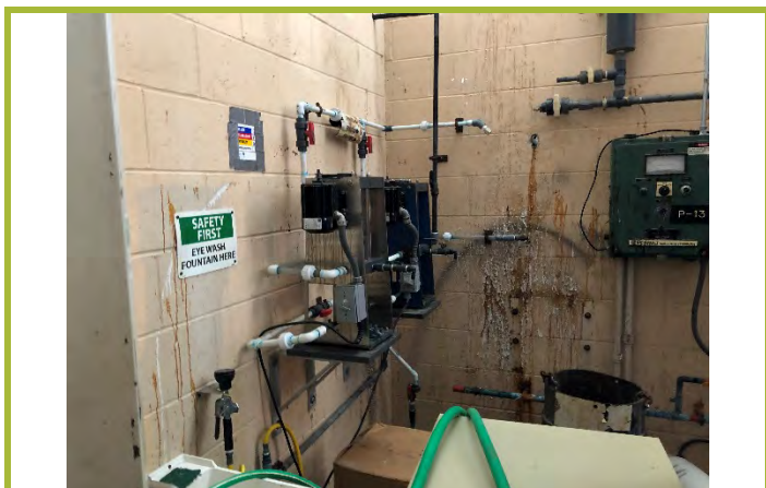
Photograph #17: Additional treatment chemical storage.
