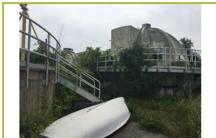
Photograph #26: Exterior wastewater treatment structures.
