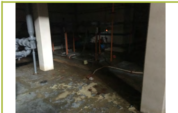
Photograph #20: Basement machine area, floor drains, and water damage.
