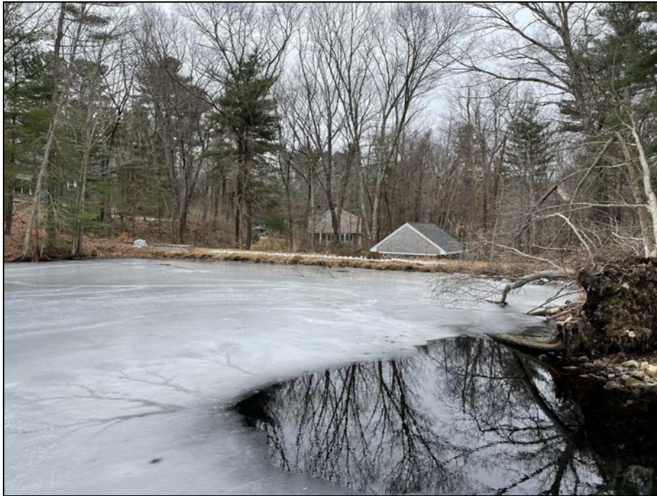
Photo No. 3.: Overview of the upstream face of the dam from the spillway approach looking downstream and left.
