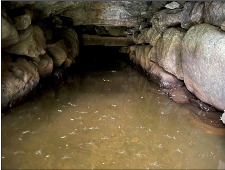
Photo No. 21.: View within the culvert from the downstream end looking upstream.
