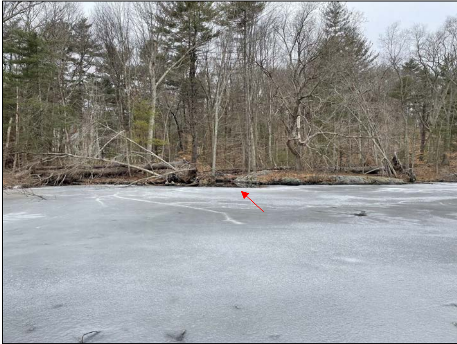
Photo No. 11.: Spillway approach (red arrow) from the upstream left abutment looking right
