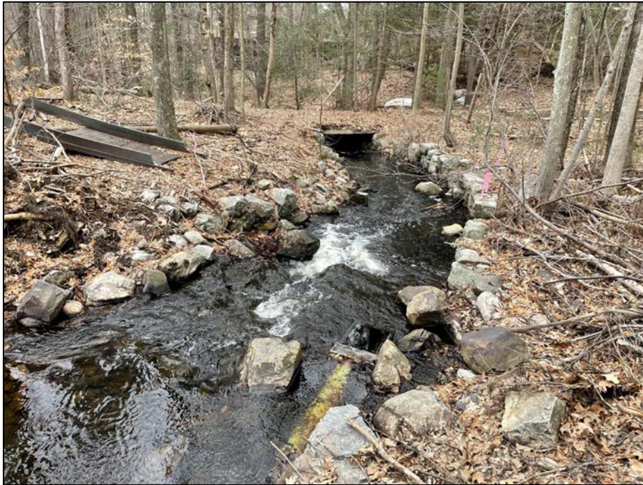
Photo No. 15.: Discharge channel of the spillway and the stone culvert from near the control section looking downstream.
