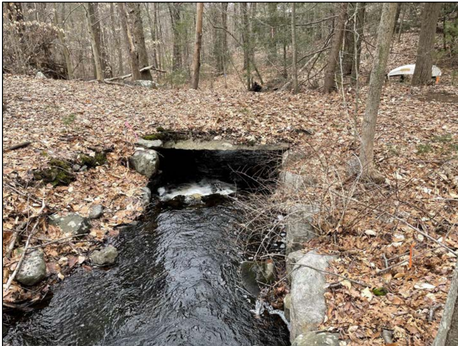
Photo No. 16.: The stone culvert that carries the spillway channel beneath the crest looking downstream.
