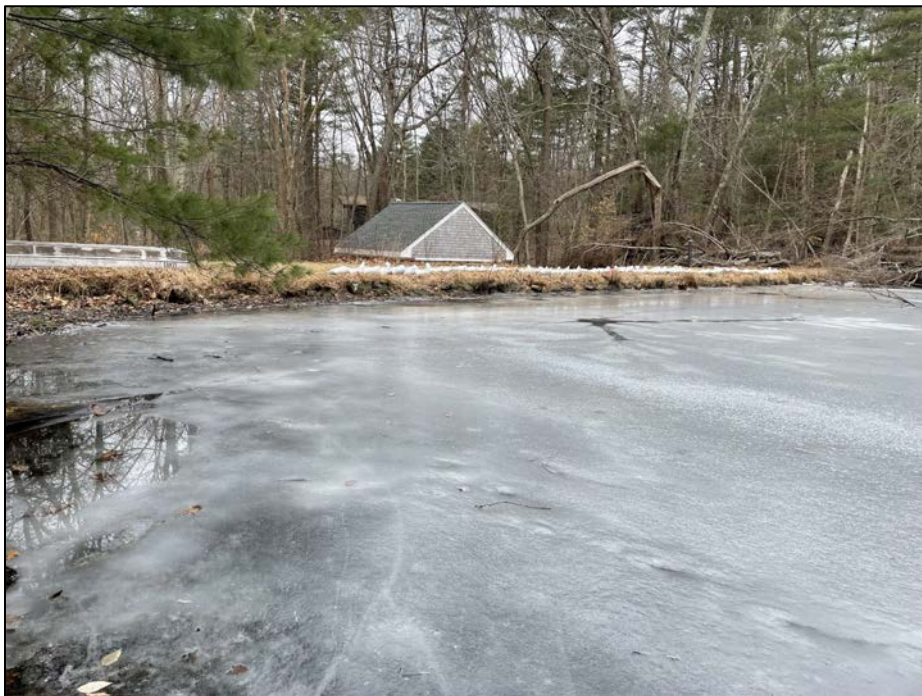
Photo No. 2.: Overview of the upstream face of the dam from the upstream left abutment looking downstream and right.
